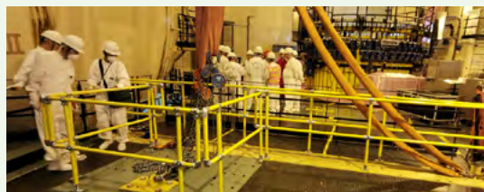
DNMC installs a guardrail on the 20m T-shaped beam in the reactor building, reducing 6 Level 1 high-risk tasks.
